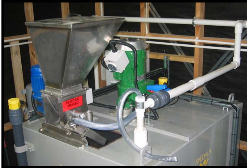
Automated Polyelectrolyte Dosing System
